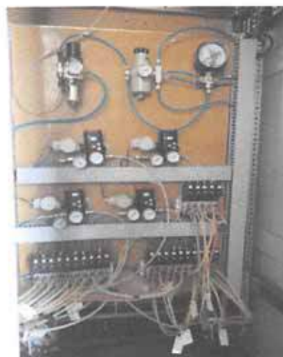
Gambar 3.1 Panel pneumatic control H2 Plant
